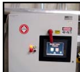
Touch Screen Mixer Control Panel
